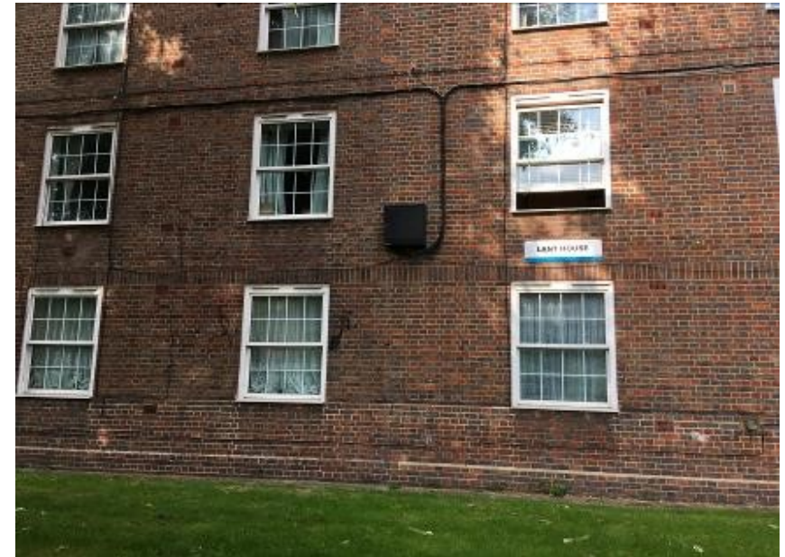
Figure 16: Inappropriate UPVC windows on Lant House, Lant Street
